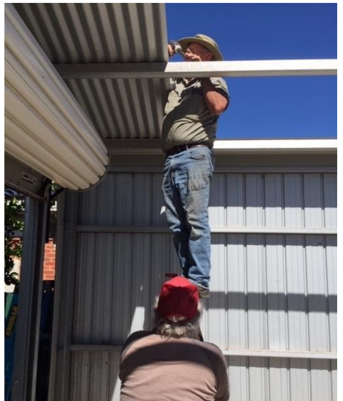
Pictured above are Barry and David dismantling the shed so it could be moved easily to the Men's Shed site.
